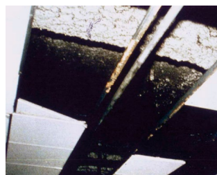
Asbestos sprayed steel beams
