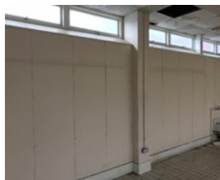
Asbestolux in a wall
