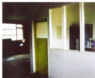
Asbestos insulating boards
