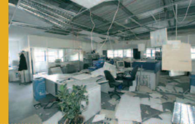
Buncefield aftermath - offices after the explosion
